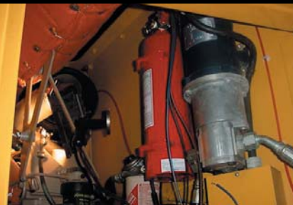
The red Firetrace cylinder can be seen here, along with the red detection tubing as it is run to the critical areas
